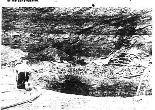
A round, concrete spillway, 11 feet in diameter, for the lake, is built in solid rock back in the side of the hill. It will carry lake water through the dam and back into Renfro Creek. The above photo shows the mouth of the spillway where the water will enter.
