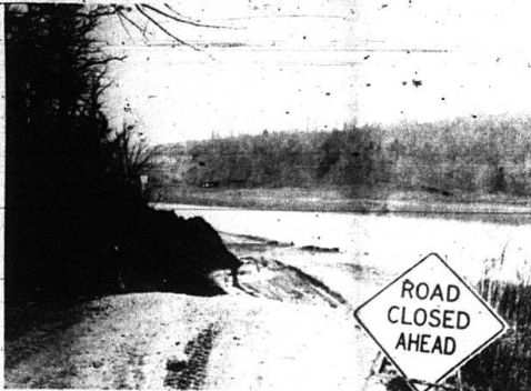
"ROAD CLOSED AHEAD" and that is exactly what the sign men's as can be seen in the above photo. The road covered in at this particular spot, just beyond the home of Mitchell Abney because it was undammed for dirt to fill the core of the dam. The State Highway Department says that it is not their responsibility to construct another road since the old road would have been covered by water when the lake is filled anyway. This cave-in causes the residents on the road to have to travel through Brindle Ridge to get to Mt. Vernon and three of the residents will be land-locked when the lake fills unless another road is constructed.
