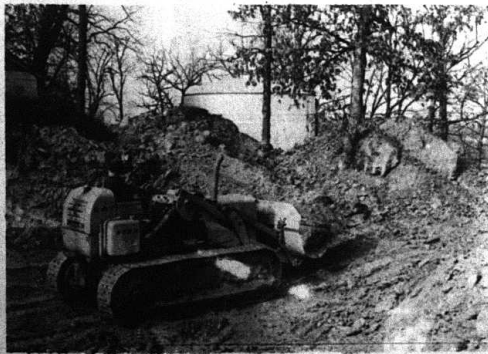
STORAGE TANK- Another 200,000 gallon storage tank and a 75,000 gallon elevated water tower will be located on town hill where the present storage tank is located. Nash and Stewart of Lexington are the contractors for the filtering plant and storage tanks.
