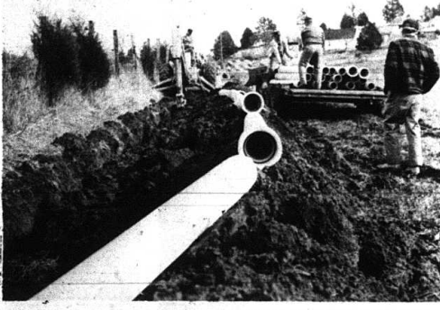
LAYING WATER LINES- In the above photo, crews are shown working on the water lines along U.S. 150 west of Mt. Vernon. About 1 1/2 miles of pipe has already been laid.
