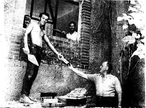
REMODELING BEGINS: The Rockcastle County Farm Bureau has begun remodeling work on their building located on old U.S. 25 in Mt. Vernon. Henry Miller, left, and Wesley Renner, are shown laying brick to close up a window in the old garage part of the building. This section of the building will be used for Farm Bureau's new Tire and Battery Program. Farm Bureau Agent William K. Bullen is shown in the photo with the workmen.
