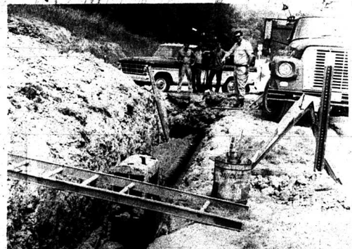
Fred W. Leath Associates, contractors for the new water line system in Mt. Vernon and surrounding areas, are presently engaged in boring holes to install water lines under Interstate-75 at Reno Valley. The pipe must be laid in a manner that, if necessary, it can be replaced without tearing up the entrance and exit from the interstate. Laying of the water lines is also about three-fourths complete.
