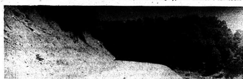
The new road around Lake Linnville is nearly complete, according to Elmo Anderson, sub-contractor for the project. Pictured above is a small section of the road which is on the west side of the lake. The Reno to Brindle Ridge Road, also newly constructed, has been open for traffic for several weeks. This portion of the new road will probably be ready for traffic within the next week.
