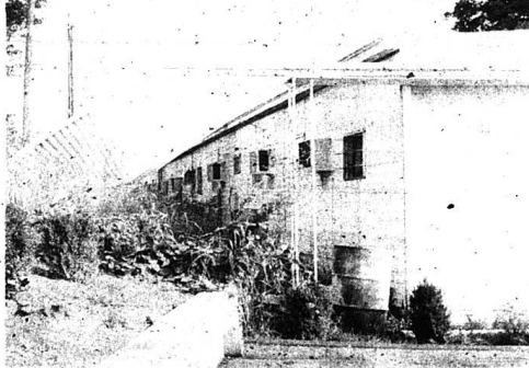
The Twin Maples Motel in Mt. Vernon was one of the structures most heavily damaged by winds Monday evening. Winds tore the awning from the front of the motel and laid it over the back of the building. Ed Winstead, owner of the motel, estimated the damage at between three and four thousand dollars.
