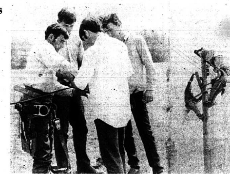
The above photo shows a Mercury Vapor Light being installed at Mt. Vernon School by the Industrial Electric Class of the Harry Sparks Vocational School. The class was able to do this job because of new equipment which was added for this year's class and because of Kentucky Utilities' co-operation with our lineman program. Students shown on the pole are Dennis Remmer and Ricky Price. Standing are, from left: Stull Philbeck, David McCauley, James Lambdin and James Phillips.
