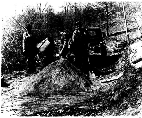
Workers at the Great Saltpeetre Cave are shown building a Coon cage near the entrance to the cave. Along with the Coon, several animals, including a Peacock, will be housed in this area as an added attraction to tourists. John Lair, owner and developer of the historic site, has already built a dam across Crooked Creek and will stock the backed up water with trout.
