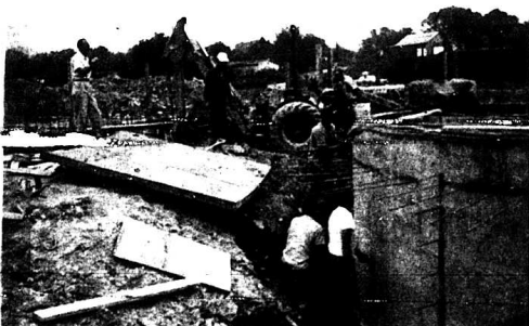
NEW SEWER PLANT-- Charles Alfred Mullins, extreme left, engineer for Crawford & Crawford Engineers, gives instructions to workers on the sewer plant under construction in the Robbins Bottoms behind the Bowder Nursing Home in Broadhead. The plant is also scheduled for completion June 1, 1972 and is being built by MacGregor and Neal Construction Co. of Lexington.
