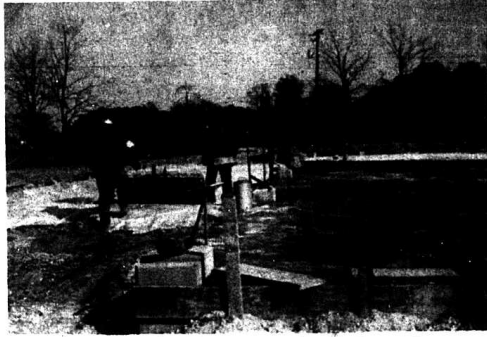
Construction on the new State Highway Maintenance Garage for Rockcastle County is well underway. R.E. Elvirine Construction Co. of Campbellsville was the successful bidder at $98,500 for the metal building which will contain 7800 square feet of maintenance garage and office space. The building is scheduled for completion by March 1, 1972. The site for the garage was purchased from Dr. J.D. Henderson, at an approximate cost of $15,000 for ten and one-half acres sited in located just off U.S. 50 south.
