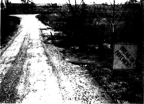
A new box culvert will replace the old one shown in the above photo on the Shirley Caldwell Road near Quail. The old culvert was washed out during September. This project falls under President Nixon's Emergency Employment Act which is a federal program designed to provide jobs on public works projects to persons currently unemployed. Salaries of the workers are provided by the government while the state pays the cost of materials and equipment. Estimated cost of the project, which is scheduled for completion by next summer, is $9,165.00.
