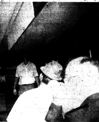
Executive Vice President Jess F. Bullock looks over the damage done by fire in a lightning fixture ballast at the Bank of Mt. Vernon last Friday afternoon. Mr. Bullock estimated the damage at $1,000. After the first call, city firemen had to return to the scene to extinguish another blaze-up in the same location.
