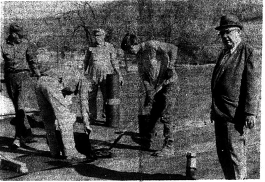
NEW ROOF-- A much needed improvement, a new roof, is presently being put on the Rockcastle County Hospital. Watching the work in progress is County Judge Charles Carter. Materials for the project were furnished by the County and the workmen through the Federal Emergency Employment Act which is administered through Judge Carter's office.
