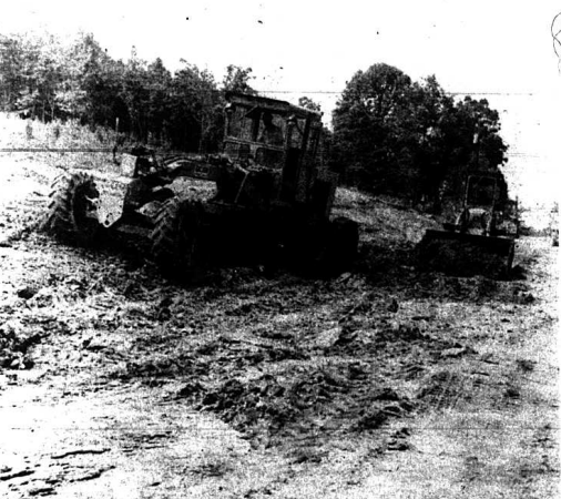
The State Department of Highways is currently repairing Town Hill Road, just north of Mt. Vernon. The state, according to Evans Hilton, district highway engineer, plans to widen the road where feasible and apply a bituminous surface for one mile. Approximately 30 families live on the road.
