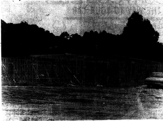
The Rockcastle County Library building is taking shape, as can be seen from the above photo. The building, which is 52.8 x 96 feet, will house an assembly room in one end, a reading room, two storage rooms, office space, two rest rooms and a kitchen. The outside of the building will be brick veneer and there will be ample parking available. County Judge Carter said he expected the building to be completed some time in the late fall. Floyd Stokes is foreman of the project for the county. The building is located on U. S. 25 adjacent to the property of Ed Winstead.
