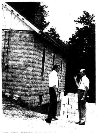
THE REV. HENRY PARROTT, Supt. of Missions for the Rockcastle County Baptist Association, right, makes a point to "Brother Joe" Mobley during construction of an addition to the Mt. Zion Baptist Church.
