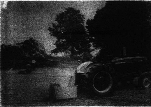
ALMOST COMPLETE —The grade, drain and seeding portion of constructing the new football field at RCBS is almost complete. The above photo shows a workman on a tractor which removes small rocks from the field while in the background, workers are covering with straw the newly seeded portion of the field.
