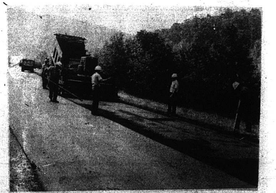
Quite a lot of blacktop is presently being spread in Rockcastle County. The above photo was taken on U.S. 25 which is being blacktopped from Mt. Vernon to Roundstone. The work is being done by Allen and Company of Winchester.
