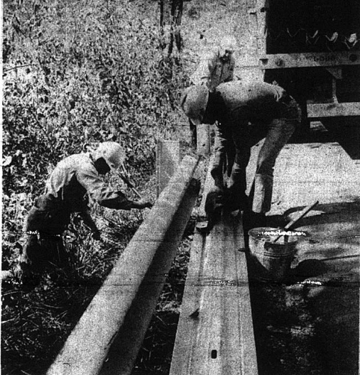
A safety feature long needed in this county was finally installed this week when workmen from the District Office of the Department of Highways began installing guard rails on Ky. 1004 (Brook Creek Road). The road runs along the side of a steep hill, is narrow and the very real danger of a car, or a bus load of children, going off the road and down the steep, long incline was ever present. According to Magistrate Ernest Mason, he put the guardrails on his list of priority improvements needed by the Department of Highways as soon as he took office.
