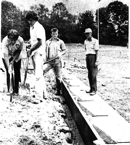
BUILDING BLEACHERS - A section of concrete bleachers are presently being built for Rockcastle County football for this year. A section, one seat high and 100 feet long, is expected to be completed for the first game. Labor for the project is being furnished by the County Judge's office, the school board and the CETA program with materials being furnished by the school board. Working on the project are, from left: Albert York, Paul Mason, Jim Wynn and Paul Owens.
