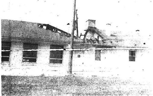
As can be seen from the above photo, the fire last Wednesday night at Mt. Vernon Elementary School began in the furnace room. The fire wall which separates the two sections of the classrooms can be seen on the right of MVES School Principal Buford Parkerson credits this wall and quick action by the Mt. Vernon Fire Department with preventing the fire from spreading to the classrooms on the right in the picture. These rooms are now being used, except for the one immediately adjacent to the furnace room, and can continue to be used since they are heated by a furnace of their own.
