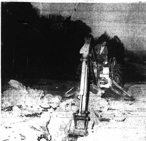
$75,000 gallons of water was lost and service was disrupted to several residents last Thursday morning following a break in the city's main water line at Belly Acres Restaurant on U.S. 52 just north of Mt. Vernon. The break was repaired quickly by employees of the city's water department.
