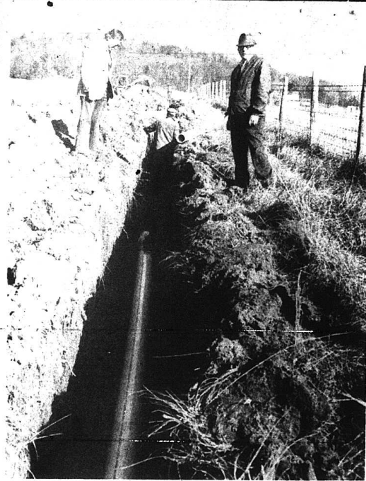
Roy Brown, president of the Western Rockcastle County Water District, left, and Robert Paul, owner of Paul's Pipeline, watch as the first pipe is laid for the water district's system. Mr. Paul's company has the job of laying over 70 miles of the line in Rockcastle and Lincoln Counties.
