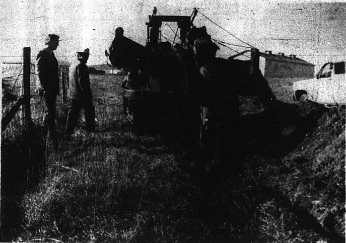
Monday, work began on laying the pipeline for the Western Rockcastle Water Association. In the above photo, Roy Brown, far left, president of the association, and Robert Paul, owner of Paul's
