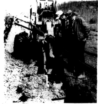
Tommy Adams, CETA employee, Rockcastle Conservation District and Junior Long, Conservation Technician, Soil Conservation Service, are shown working from the installation of the Jack Upcan farm. There were 3,800 ft. of tile installed on the Upcan farm. Other installers recently included Jim Cox, 4,000 ft.; Sherry Adams, 2,500 ft.; De William Adams, 2,200 ft.; George Hardin, 2,000 ft.; R.R. Wolfe, 800 ft.; Bill Coffey, 1,800 ft. and Eddie Norton, 3,300 ft. Assistance in planning, layout and installation was provided by the Soil Conservation Service in cooperation with the Rockcastle Conservation District. (Soil Conservation Service Photo by S.T. Vanover)
