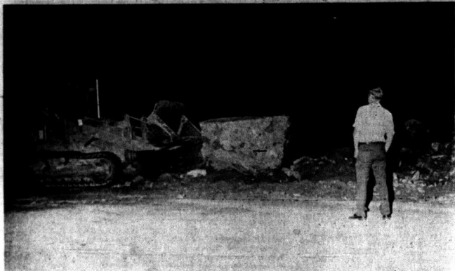
SERVICE TO KU CUSTOMERS was interrupted and U.S. 25, south of Mt. Vernon, closed to traffic for a time last Friday night when a construction crew set off a blast at an excavation site on the property of Reuben Hammonds. Gerald Thompson, KU Manager, said Monday that a double circuit (7.2KV and
