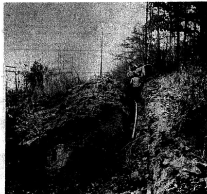
Employees of Paul's Pipeline of Danville are shown laying more water line in the Pine Hill area for the Western Rockcastle County Water District. The project is about 80% complete at present, according to Roy Brown, president of the association. Some customers in the Quail section of the county have already begun using the water.
