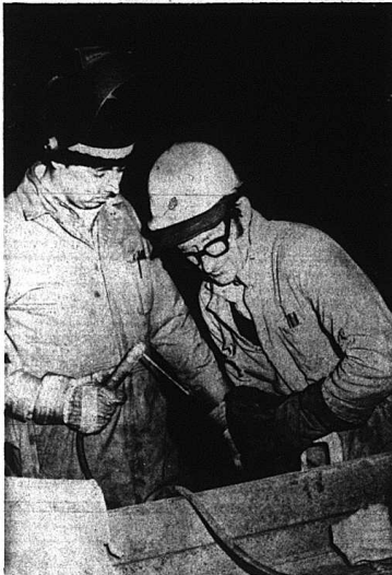
David Shivel, left, and Curtis Smith are shown putting together a truss to be used in the roof at Keeneland Race Track in Lexington. The trusses weigh
