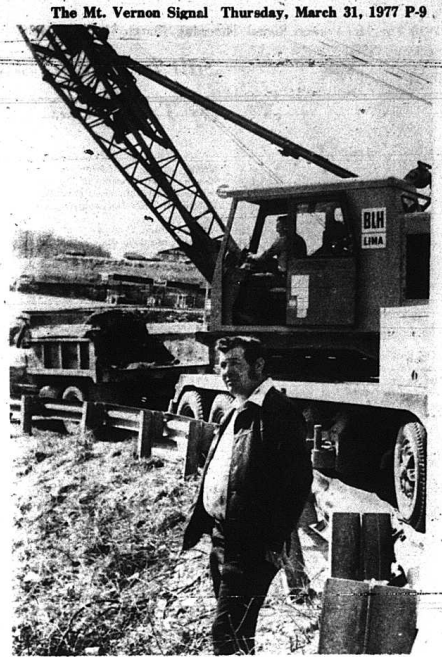
5th District Magistrate Ernest Mason looks on as fill work began Tuesday on widening of the Brush Creek Road. The curve near the U.S. 25 intersection will be widened approximately 10 feet by using a retaining wall on the east side. Work on the project should be completed within the next two weeks.
