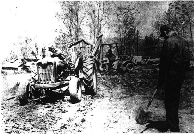
Residents in Owens Subdivision will soon be benefiting from an extension of the city's present sewer system. Several problems with septic tanks have been encountered in the area in the past
