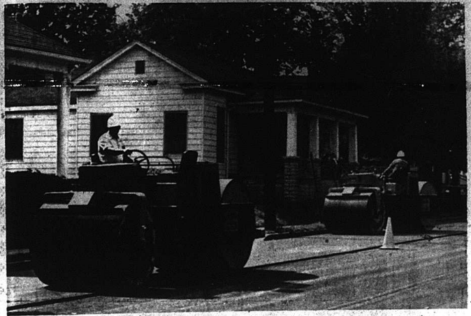
Black-topping on Richmond Street interfered with traffic last week, as flagmen directed cars into one lane. The work should be finished soon.
