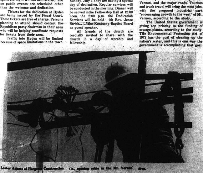
Lester Adams of Hargetts Construction Co., splicing cable in the Mt. Vernon area.
