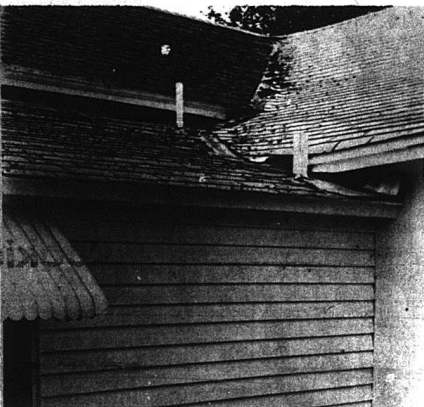
Mary Johnson's roof was damaged like this in the hailstorm.
