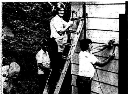
One of the three crews of workmen who are making repairs on homes. Here Russell Blackburn, Ellis Kirby and Larry Hensel work on siding for a house near Livingston.
