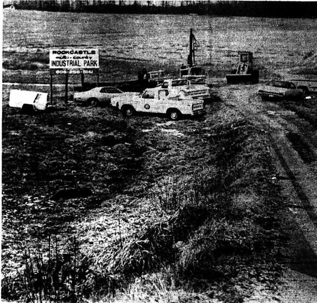
Construction has started at Rockcastle Multi-County Industrial Park near Mt. Vernon. Mays Construction Company is now laying water and sewer lines, and some of their equipment is shown above.
