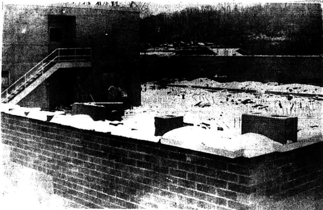
Snow has stopped construction of the Skilled Care Facility at the Rockcastle County Hospital, although workmen were able to get the ground level walls up. Lower level will contain physical therapy department; upper level will be rooms for patients requiring skilled nursing care. Working is being done by Browning Construction.
