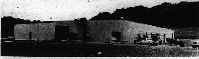
Almost finished—The Rockcastle Manufacturing Company stands in the Industrial Park today with a completed exterior, but about a month's more work needed on its interior. Access roads have been completed.
