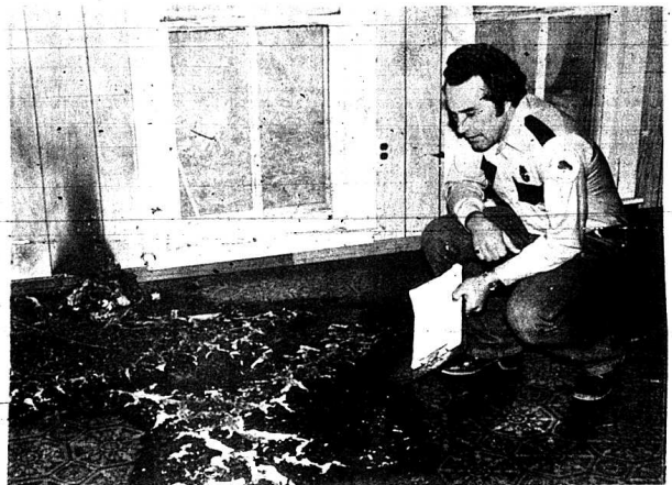
While on the scene, the fire department inspected an uninhabited house on the property and found evidence of an arson attempt in one of the rooms in
