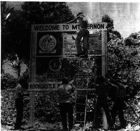
City employees and CETA workers were busy last Friday erecting signs at the entrances to Mt. Vernon. The signs hold the symbols of all the local civic organizations and, in the center, also holds the sign Mt. Vernon received for being designated
