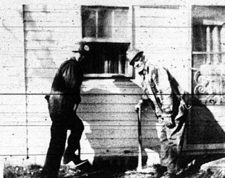
A COLD WINTER Sun was shining over the home of Minnie Sutton, Broadhead, when Green Thumbers Ames Bowman and Ben Cox began work underplanning her home. The men work as part of a weatherization crew through Community Action to help winterize homes of low-income elderly.
