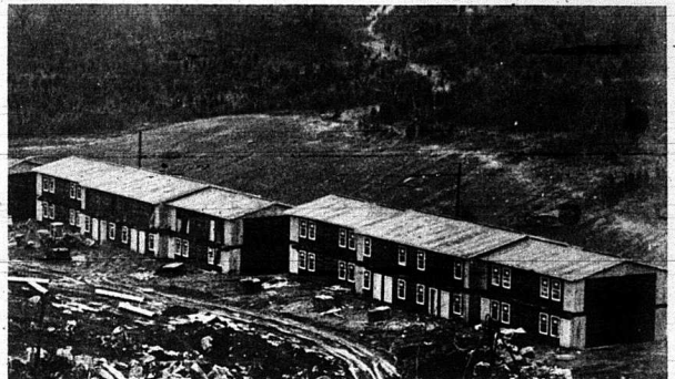
Construction is progressing smoothly on the low-income government subsidized housing units Valley View Apartments being built off old U.S. 25 South by Lovins Construction Company of Somerset. The 32-unit one, two and three bedroom is co-owned by Jerry Ikard. Completion is set for Spring of this year.
