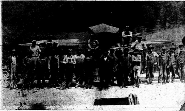
The above picture was taken in May, 1931 (during the depression) and shows those lucky enough to be employed. The men were state highway workmen and received 20 cents an hour or $2.00 a day for their labor. The picture was taken on old U.S. 25 above the old Winstead Camp by Theopolis Figg. Left to right (front) are, Clell Pike, Albert Hickey, Ed Owens, Joe McHargue, Steve Gab-
