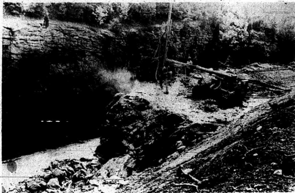
U.S. 25 is barely visible to the left in this picture taken of work being done on the rock overhang in the cut south of Mt. Vernon. O.V. Ridner, superintendent of the local job for Melco-Greer
