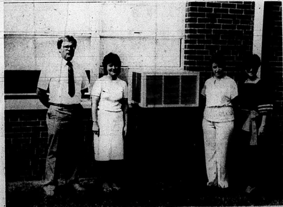
Members of the Roundstone P.T.O. Air Conditioning committee are shown above with one of the eighteen new units purchased for the grade
