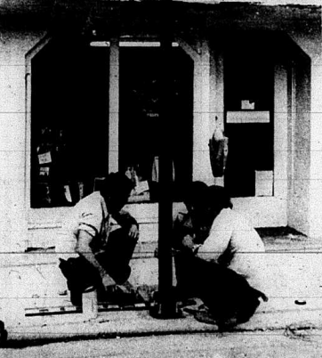
New Streets Lights . . . The City of Mt. Vernon in conjunction with the local development corporation recently installed 25 new street lights on main street. Shown above installing one of the lights are city employees, Burgess Mullins, Dennis McClure and Jimmy Rickels.
