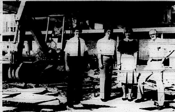
Construction is underway on the new remodeling last Wednesday are Keith Smith, Violet Cash, Delores Phelps and President Bobby Proctor. During the addition is slated to finish around the first of the construction the drive-in window will be closed but year. Employees looking on during ground breaking the lobby will be open until 6 p.m. on Fridays.
