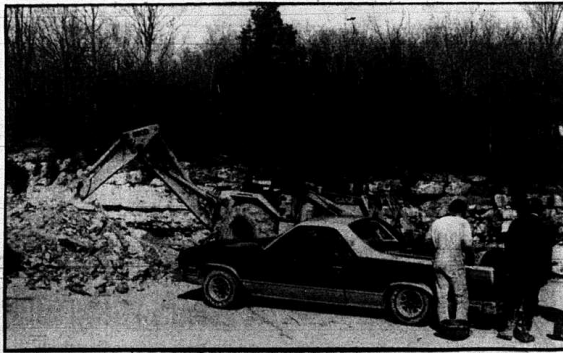
MOVING AROUND -Workers for Smith Contracting of Lawrenceburg prepare to move a Mt. Vernon Water Works water line across U.S. 25 near Vern
