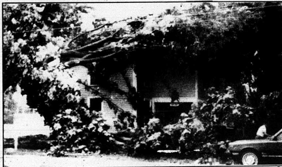
HOUSE DAMAGED —A strong wind about 4:15 p.m. last Thursday blew a large tree on a house belonging to Dwight Griffin near Mt. Vernon Elementary School. The roof of the house was
