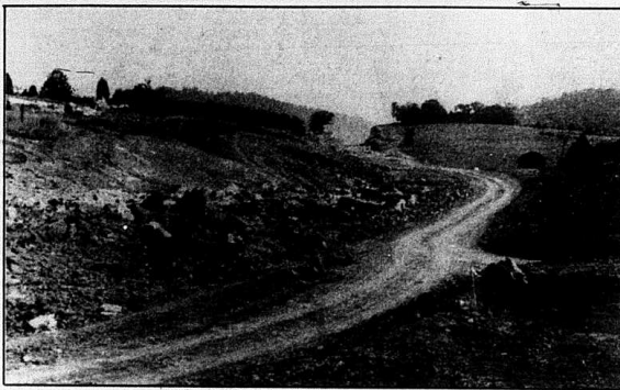
HIGHWAY WORK PROGRESSES —Work is progressing well on section of new KY 461 west of Mt. Vernon. The section is between U.S. 150 and Wadd. Bids on other sections of the highway remain right-of-entry.
