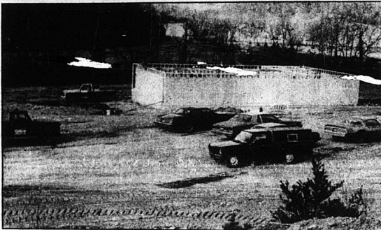
New truck plaza under construction on the I-75 Renfro Valley interchange. The picture above shows the old Valley Drive-In Theater projection booth and snack bar that has been torn down. Owner Ron Jones is standing at right in the picture. The lower picture shows the amazing progress of the plaza five days later.
