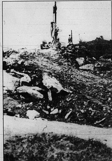
High on a hill, a workman drills a hole for dynamite as work continues at a rapid pace on the Mt. Vernon bypass of KY 461. The drilling in the picture is being done near where the new highway intersects with the old Brodhead Road.
